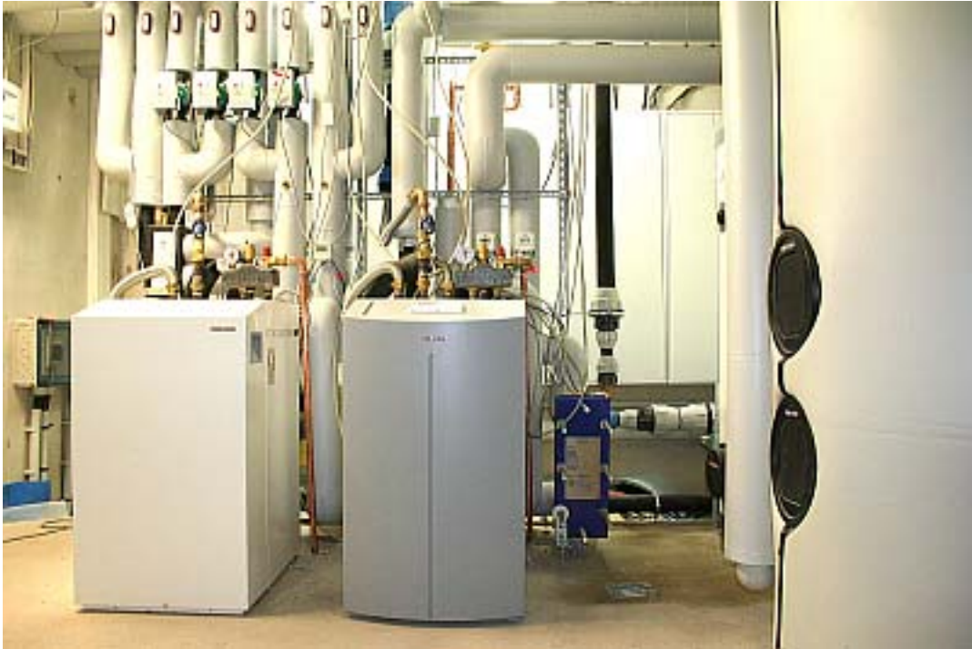
Photo 3: Two brine-to-water heat pumps (using ground water indirectly) and buffer storage
